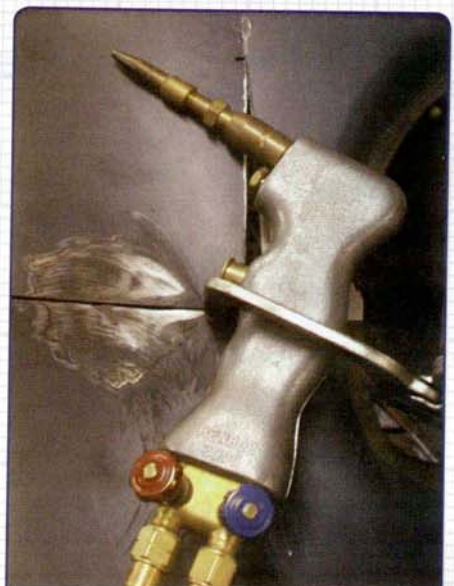
Since starting to use the modern technology gas-welding torch Dik's become somewhat of an ambassador for the product and has even been using it for lead filling. Check it out at www.welddownunder.com
